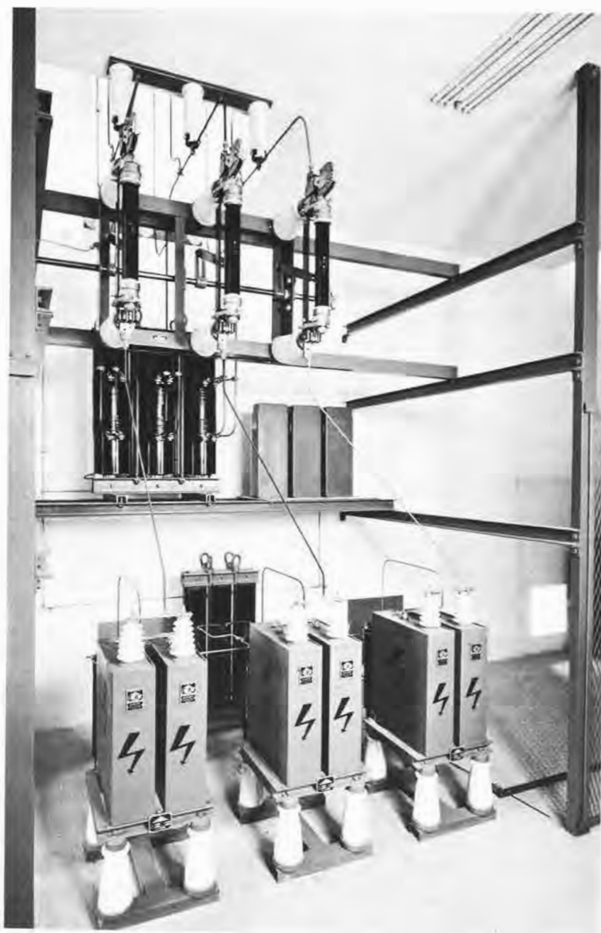
Tonfrequenz-Anlage in Mess-Station
